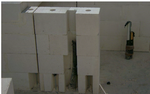
Picture demonstrating the U shape recessed into the wall with plumbing pipe
