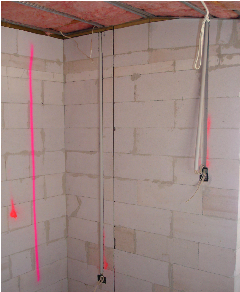
Photo of conduit being installed in chases cut in wall after construction
